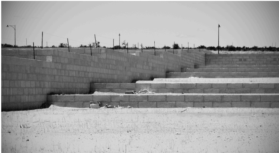
Figure 5. 12 ft (3.5m) high retaining walls in preparation for residential subdivision in northern Perth. Indigenous remnant heath vegetation and natural topographic landform is visible in the background.
